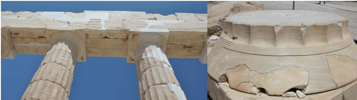
Fig.2: The columns of the Parthenon (left) employ a dry-assembly, interlocking system where wooden pins are placed in the central alcove of each drum (right) to align the structure. Overall stability is ensured by the own weight of the structure.
