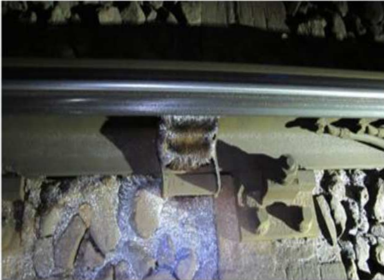
Figure 2. Severely worn narrow radius track section with wear debris at ballast and collecting magnet.
