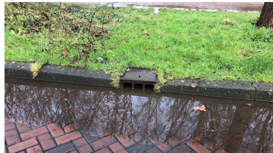
(b) Clogged filter bag in the vegetated area
