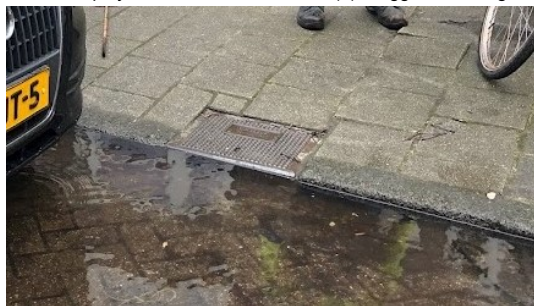
(c) Clogged filter bag in the residential area
