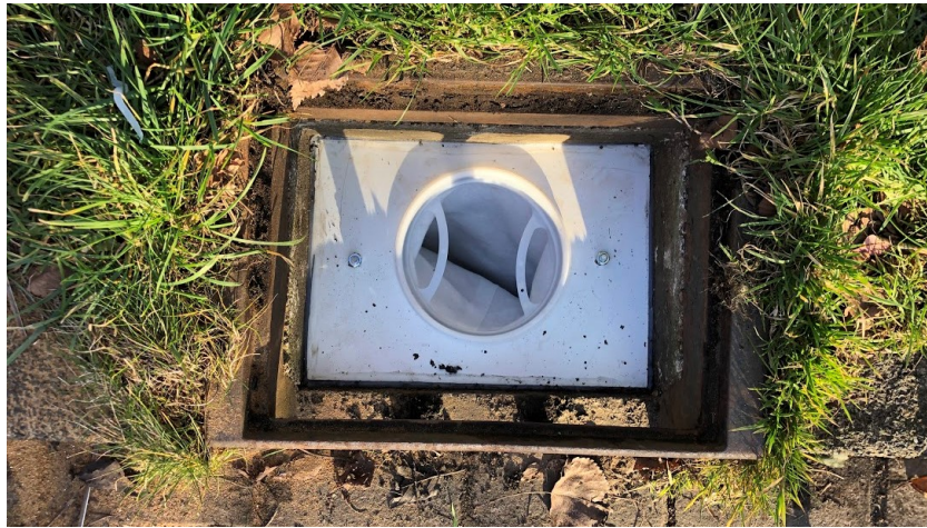
Figure 4.4: Filter bag secured in a gully pot in the vegetated area
