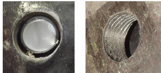
Fig. 16. Observed damages (P15.1-1)
