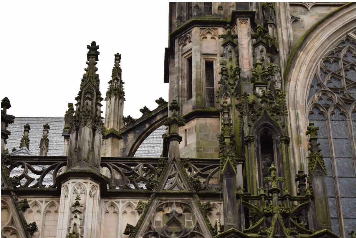
The top flying buttress on the west side of the south transept, crockets visible.
