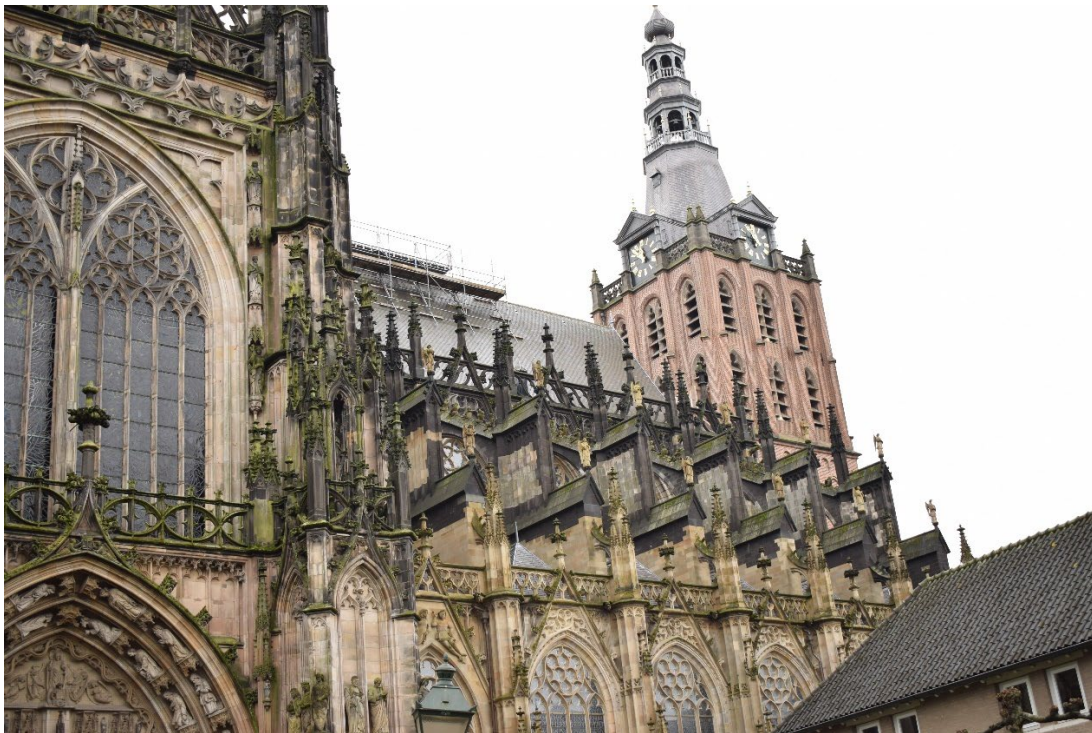
Northside of the Nave with the flying buttresses and flyer chairs and part of the north transept.
