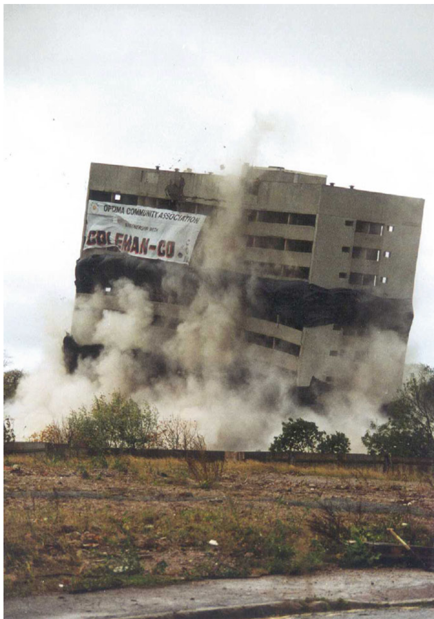
Fig. 6.7 Explosive demolition of Haddon Tower, Lee Bank, Birmingham. Source Birmingham Library Archives and Optima Community Association, used with permission
