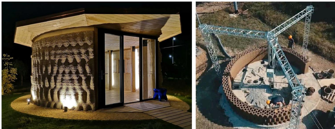
Figure 12. Gaia 3D Printed House by WASP During Construction and After Completion Source: (WASP, 2018)
