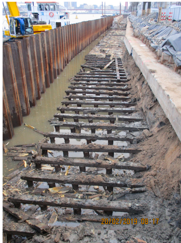
Fig. 2. Excavated historical quay wall, 'Maaskade' in Rotterdam. Photograph: Julianus, Eric. "Exposed timber pile foundation of the Maaskade". 2019. Havenbedrijf Rotterdam.
