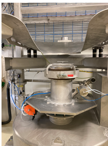
Figure 2.7: Small silo beneath bigbag tipping station at Nestlé
