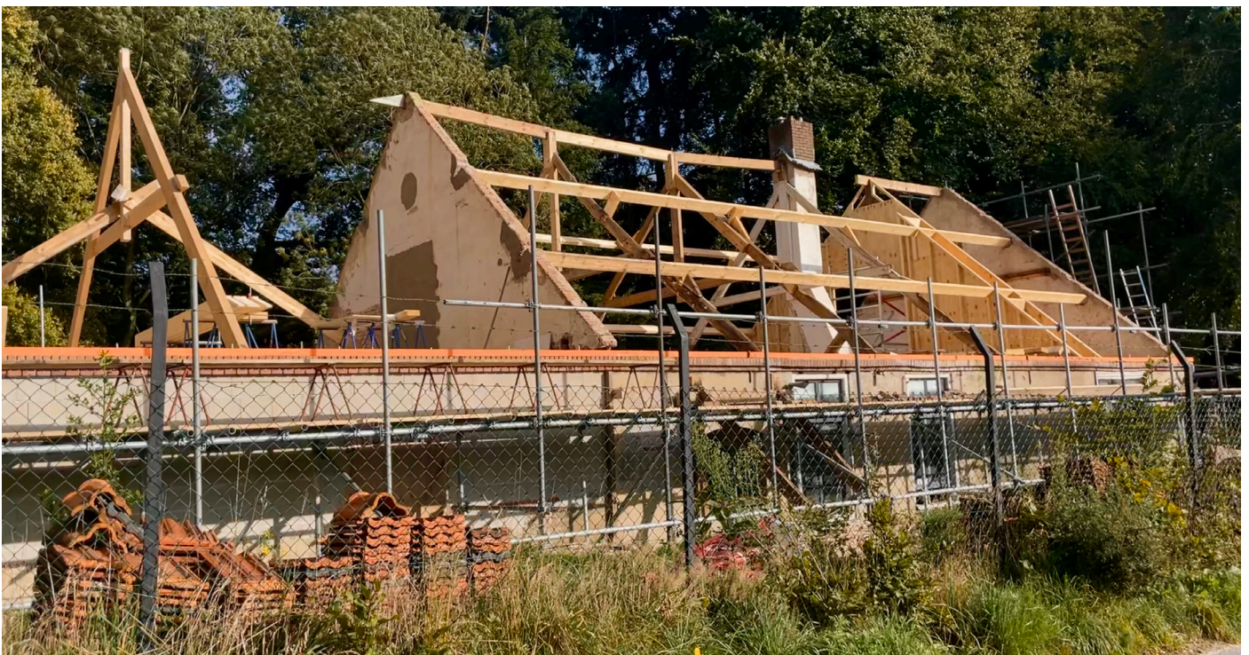
The Nederrijk area, renovation of roof structure of farm on Watermeerwijk estate (By author, 2023)
