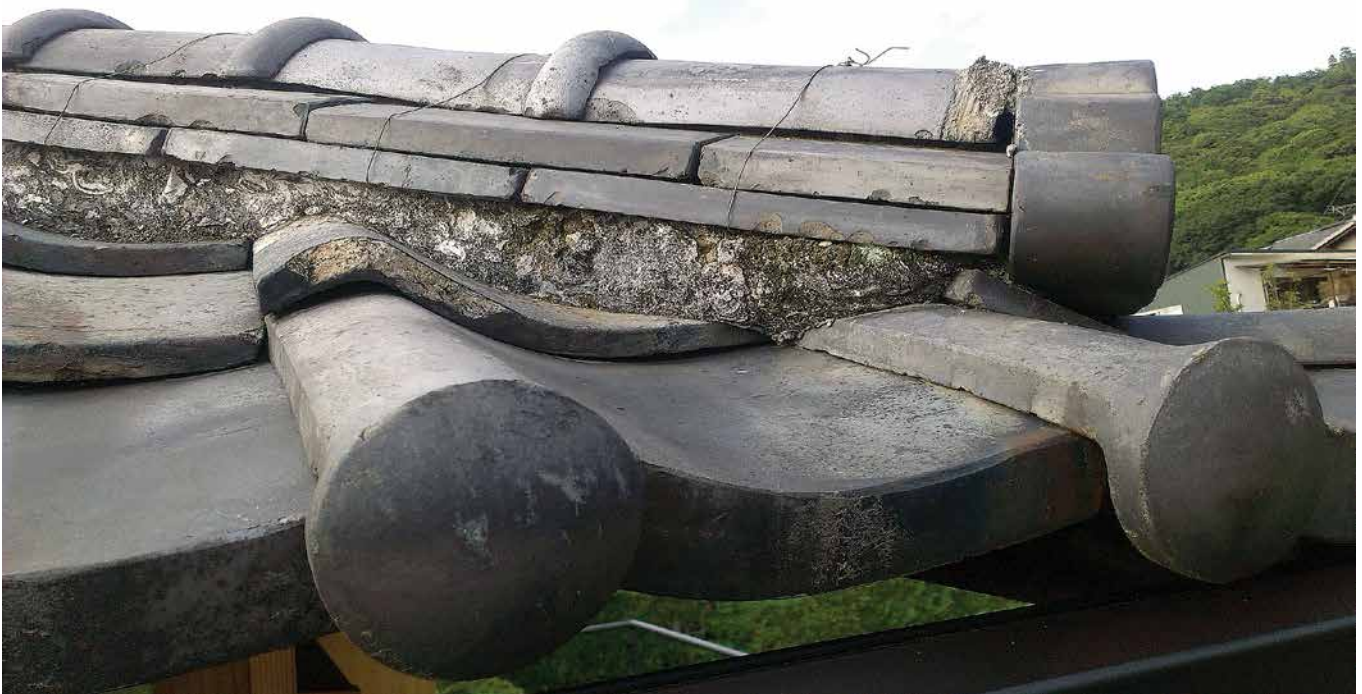
FIG. 19 The ridge of a roof in a recently restored machiya: roof tiles are laid on a bed of clay, lime and straw
