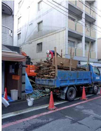
FIG. 18 A machiya pulled down and deported (2015)
