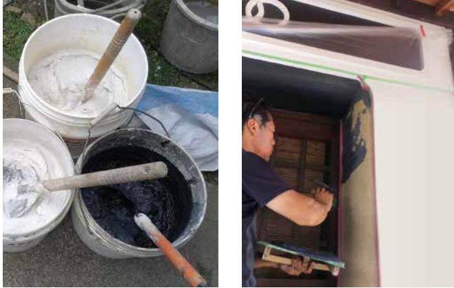
FIG. 11 White and black shikkui and its application on the exterior of a kura building (sakan from Mr Hagino's company)
