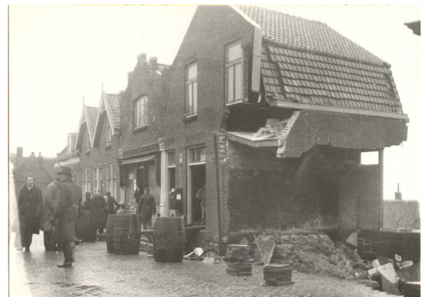
(b) Failure of external walls in Zwijndrecht during the 1953 flood (Historische Vereniging Zwijndrecht)
