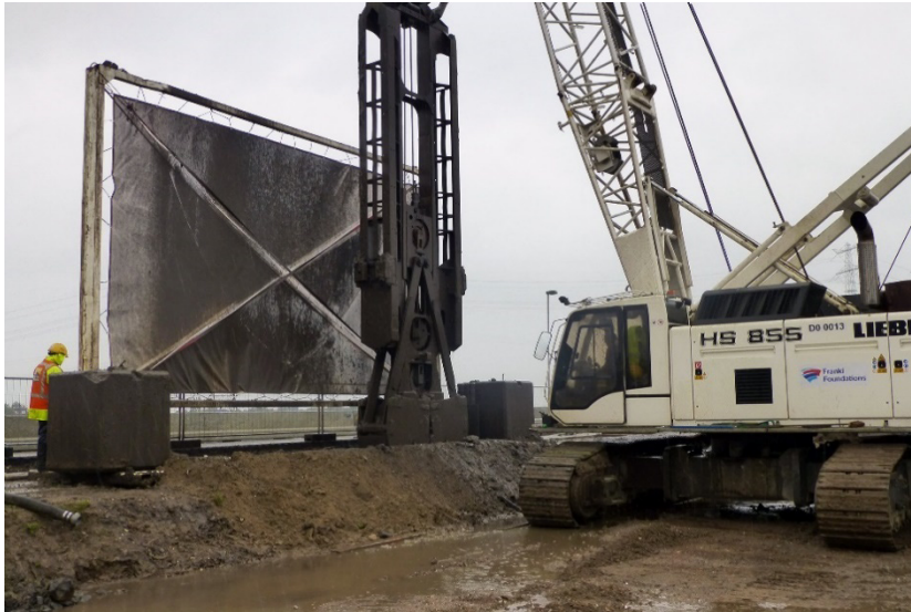
Figure 14: Installation of a concrete diaphragm wall near the outer edge of the embankment crest with a grab trenching machine, near Schoonhovenseveer, Netherlands.
