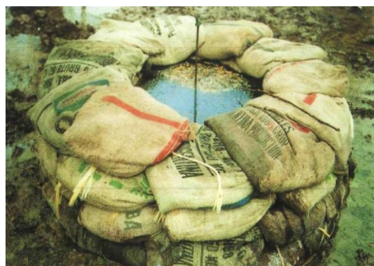
Figure 2.3: A boil ringed with sandbags (TAW, 1994)
