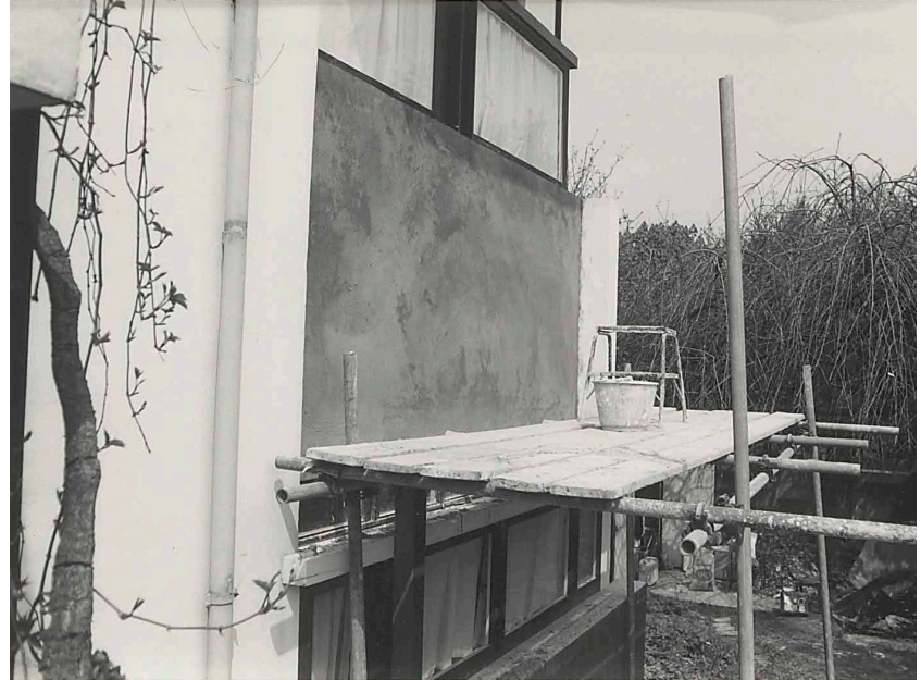
FIG. 1.11 After the plaster with hairline cracks was removed, the new render was applied in a single homogeneous coat
