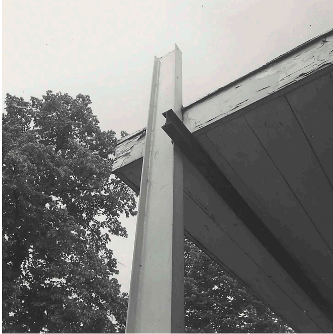
FIG. 1.4 Unconventional constructions made the house vulnerable
