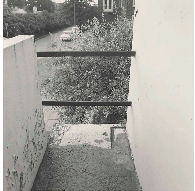
FIG. 1.5 After 50 years the concrete of the balconies also showed signs of cracks and damage
