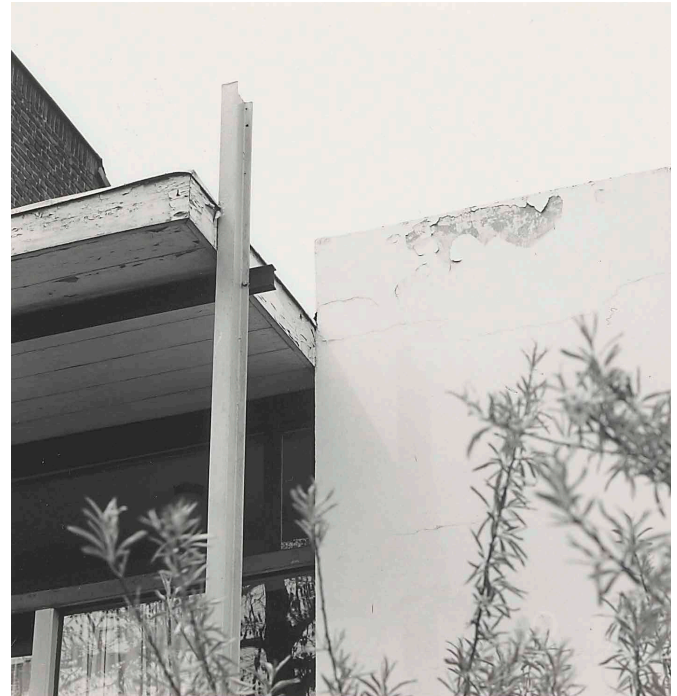
FIG. 1.3 Plasterwork and wood exhibited serious blemishes
