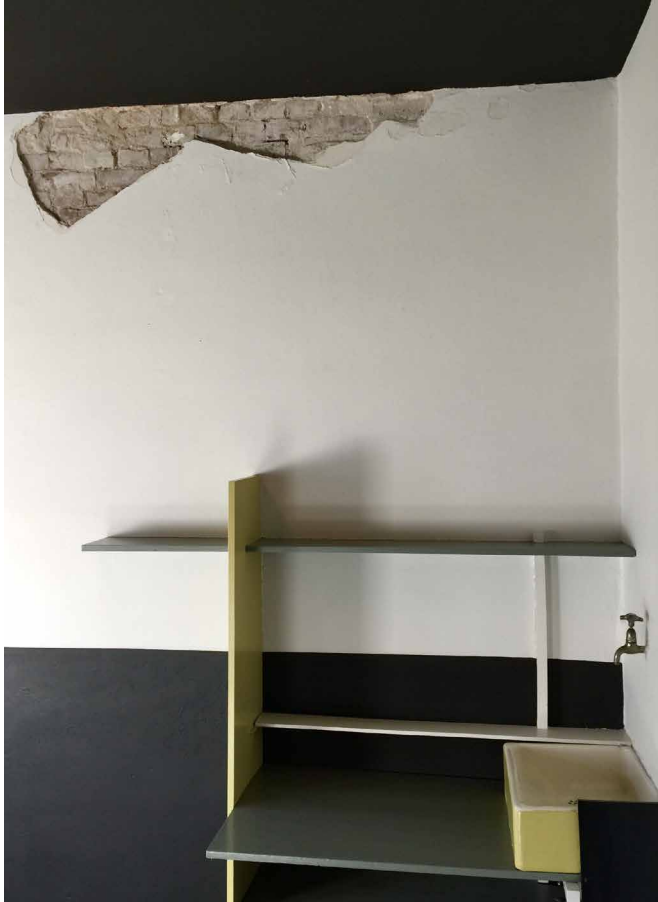
FIG. 3.13 The plasterwork at the top of the south wall of the study was damaged and came loose in October 2016
