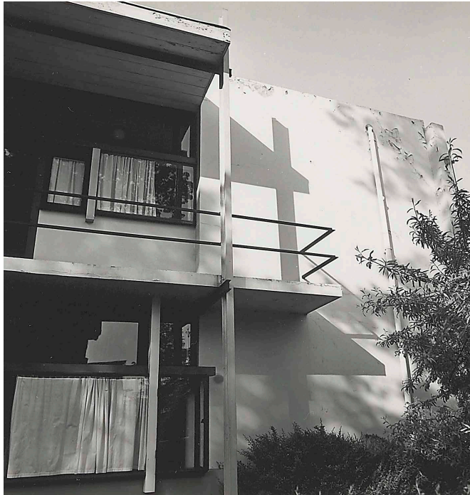
FIG. 1.2 Damage to the house became increasingly visible
