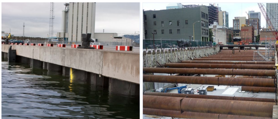
(a) Concrete cope beam on a Quay wall (picture from: Dawson Wam piling)
