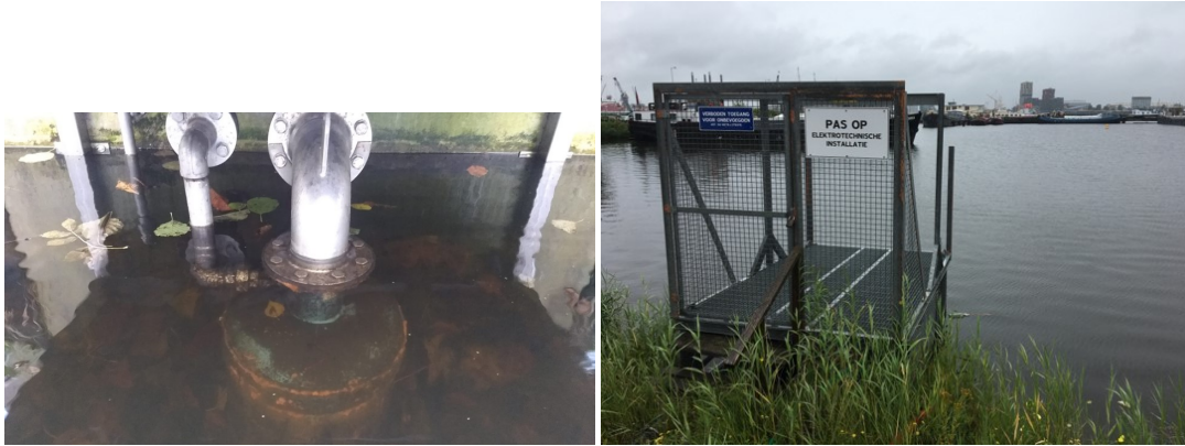
(a) Radial intake screen of SWH installation in city canal of Wageningen (b) Example of layout of a SWH system seen from waterside, Houthavens, Amsterdam.
