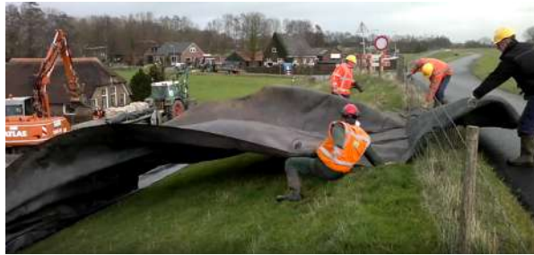
Figure 9.11: Placement geotextile inner slope during exercise water board Drents Overijsselse Delta (Drents Overijsselse Delta, 2011) during relatively windy conditions 5 Bft (8 m/s) measured at De Bilt (KNMI, 2018) (7 December 2011).
