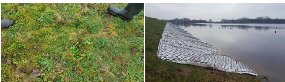
(a) Damaged grass revetment by Engerlingen , hardly any roots present. (b) Grass revetment reinforcement at the Vecht river dike near Zwolle.
