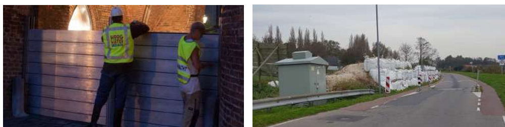
(a) Temporary flood defence Kampen (Drents Overijsselse Delta, 2017c).
