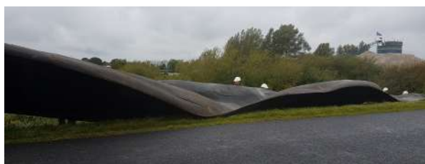
Figure B.9: Placement geotextile outer slope during exercise NATRES and water board Drents Overijsselse Delta during relatively mild wind conditions 2 Bft, 1.8 m/s measures at De Bilt (KNMI, 2018) (16 September 2017).
