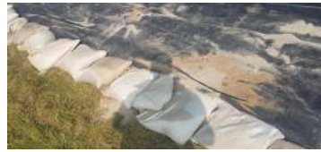
Figure 5.5: Damaged sand bags.
