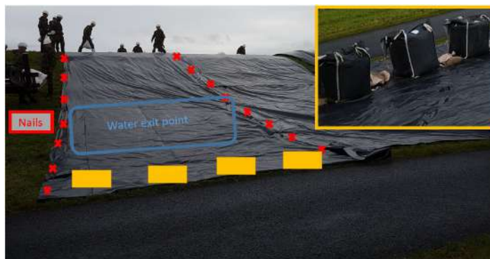
Figure C.3: Influence inner slope reinforcement measure on exit water. Impermeable geotextile loosely present at the water exit point. Chance of blocking the water and therefore raising the phreatic level in the dike is limited.
