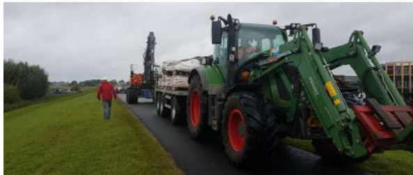
Figure 8.3: Transport and unloading at placement location during exercise at the Drents Overijsselse Delta water board (16 September 2017).
