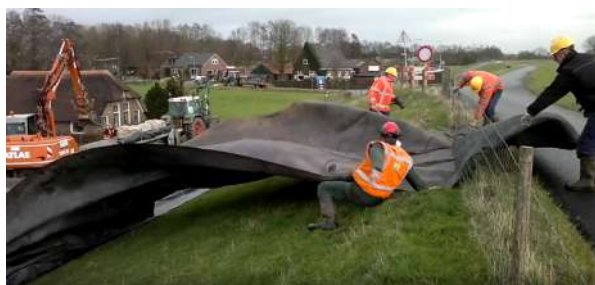
Figure B.10: Placement geotextile inner slope during exercise water board Drents Overijsselse Delta (Drents Overijsselse Delta, 2011) during relatively windy conditions 5 Bft, 8 m/s measures at De Bilt (KNMI, 2018) (7 December 2011).
