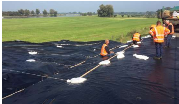
Figure B.3: Grass revetment reinforcement placed by water board Rijn en IJssel (Huijskes, 2017)
