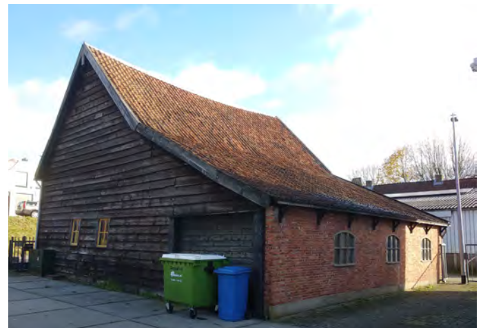
Figure 7. The western and southern facade of the barn in Oostendam. The stable post is visible between the bargeboards.
