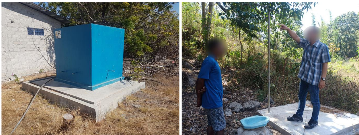
Figure 1. Examples of unsustainable WASH services in East Sumba. Left: A not functioning water tank; Right: An unfinished latrine construction. Pictures were taken by the first author.
