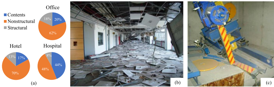
Fig. 1 a Typical distribution of structural and non-structural parts of buildings (modified after Taghavi and Miranda 2003). Damage to NSCs in Santiago International Airport, Chile, after the 2010 Maule earthquake: b damaged ceilings; c damaged lift motor (pictures from Cowan et al. 2011)
