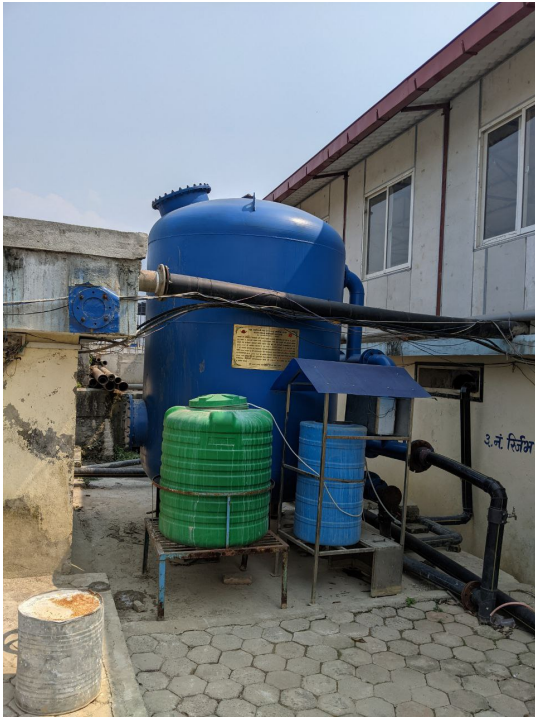
Chlorine storage and mixing site
