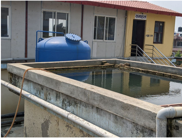
Sand and Gravel filter (before chlorine)
