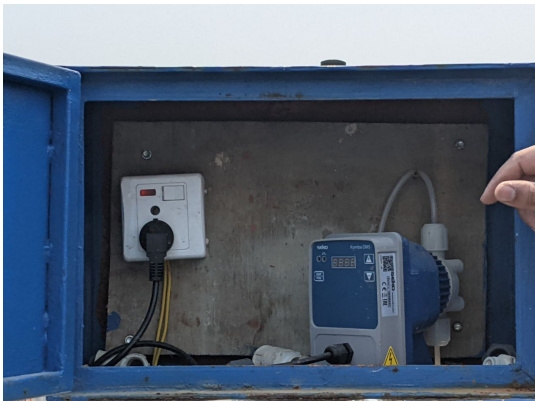
Automated chlorine dosing pump
