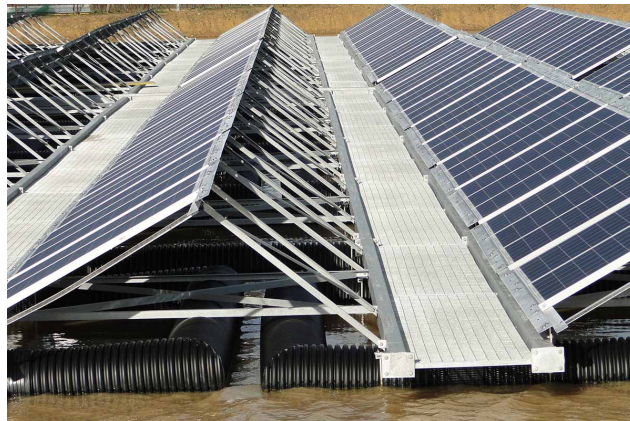
Figure 2.1: Tubular float system installed by Terra Moretti [5].
