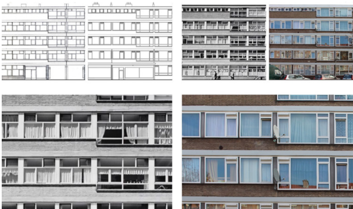
Fig 12. Replacement of window frames without considering the heritage value of the former frames (Havinga et al., 2020)
