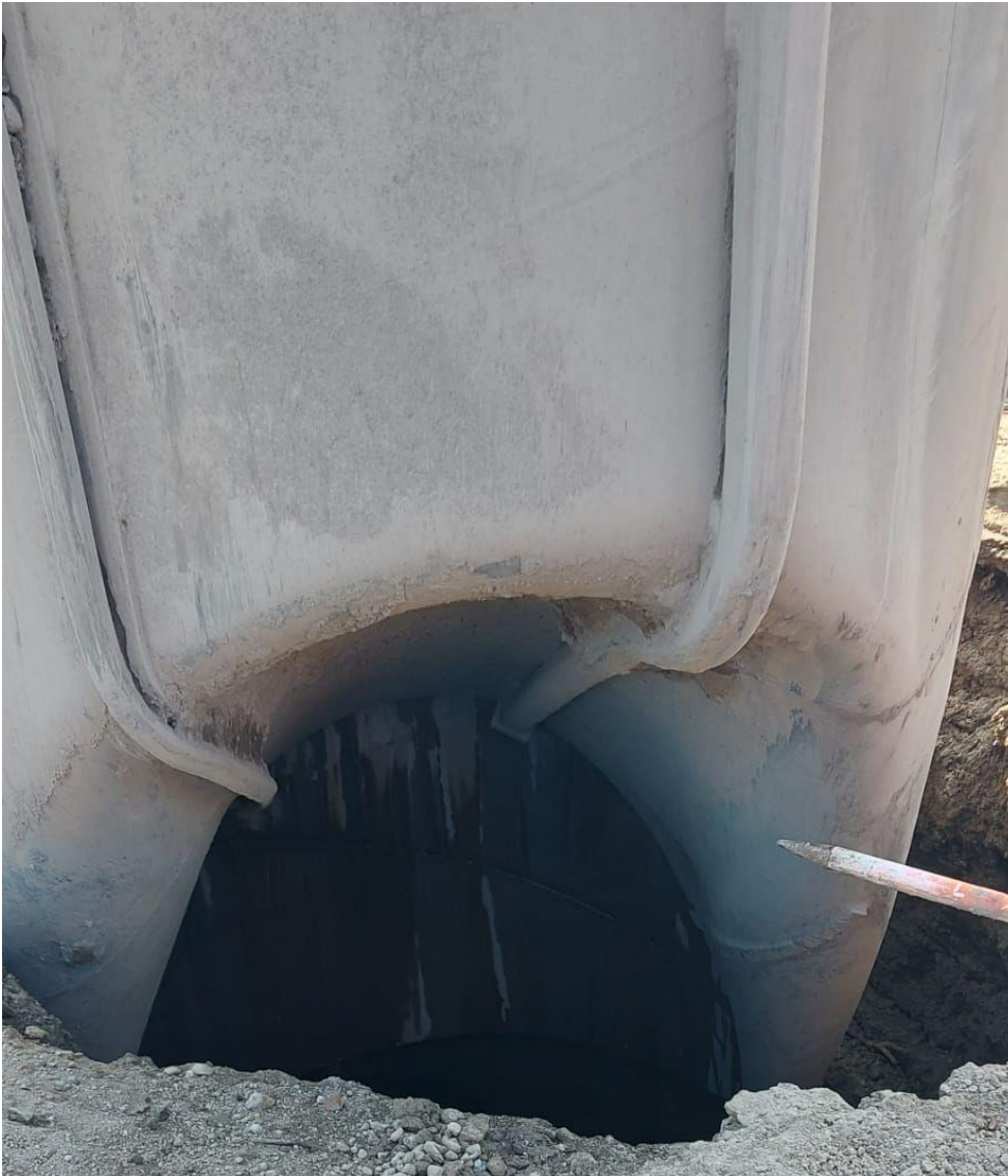
Figure 7 The foundation pile after the test shows the deformation (Witteveen en Bos, 2024).
