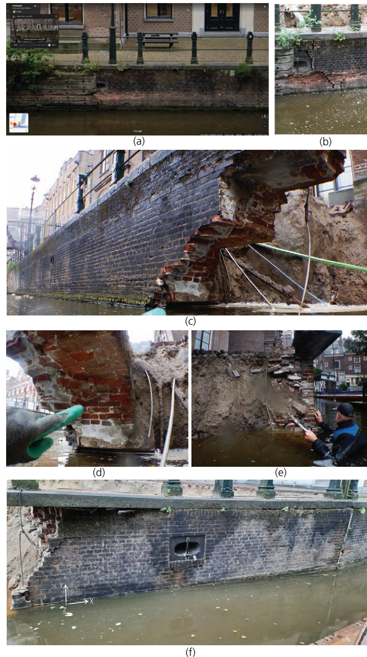
Figure 3. Cracks in the quay. (a) Ship collision crack ref. 2 from Google 1 year before collapse. © Google. (b) Crack B visible minutes before the collapse. (c) Eastern crack ref. 3 after collapse. (d) Eastern crack ref. 3 detail with sharp surface in bricks. (e) Western crack C after collapse. (f) Front view of western crack ref. 1 left and dilation joint ref. 5 on the right
