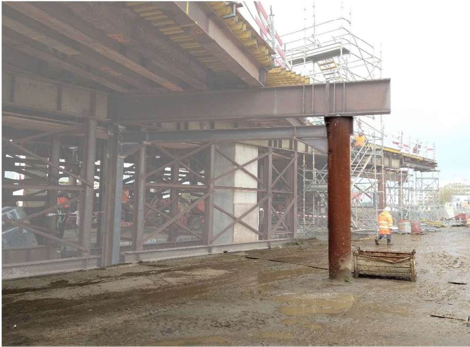
Figure 6 Picture of the case study; a steel foundation element (highlighted). The case focusses on the width, depth and koppejan calculation of the pile. Also the load and position are variables of the pile in the variables of the case study.
