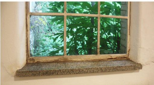
fig. 6.56 Rust on steel window frames of the ordinary barrack (20 sept 2016)
