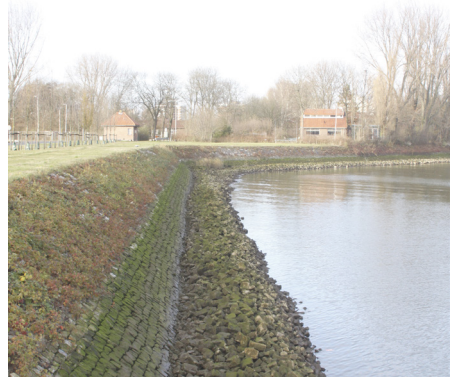
fig. 3.9 Sloping stone quay at the dike towards the quarantine area (M. Bijkerk)
