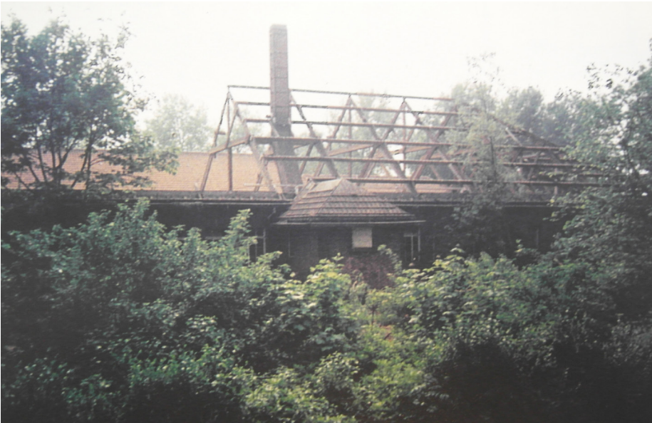
fig. 6.28 Roof construction visible during the demolition of the contact and captains barrack in the 1990s, seems to be in quite good state. (Source: Initiatiefplan Quarantaine inrichting Beneden Heijlplaat. (1997). Vereniging tot Behoud en Beheer van de Quarantaine-inrichting)
