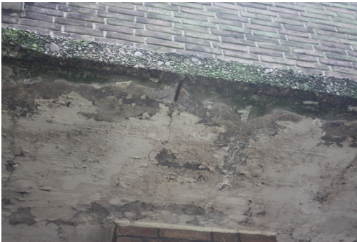
fig. 6.54 Damages on concrete canopies (20 sept 2016)
