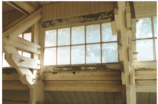
fig. 6.55 Wooden windows inside the disinfection building, showing decay of the paint (20 sept 2016)
