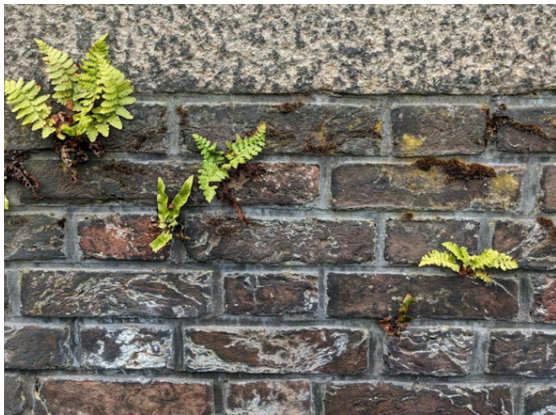
Figure 47. The wall of my apartment building.
