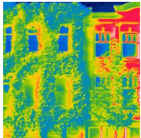
Figure 2.23. Facade covered by Boston ivy taken with ifrared camera in summer shows that the temperature of the vegetation is less than the bare wall (perini et al., 2011)
