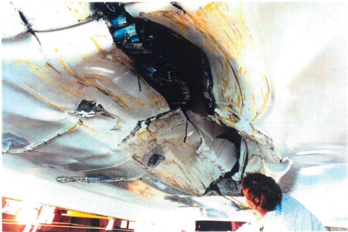
Figure 17 Part of the damage path to the bottom structure of the test-section. Failure mechanisms visible: folding, denting and tearing.
