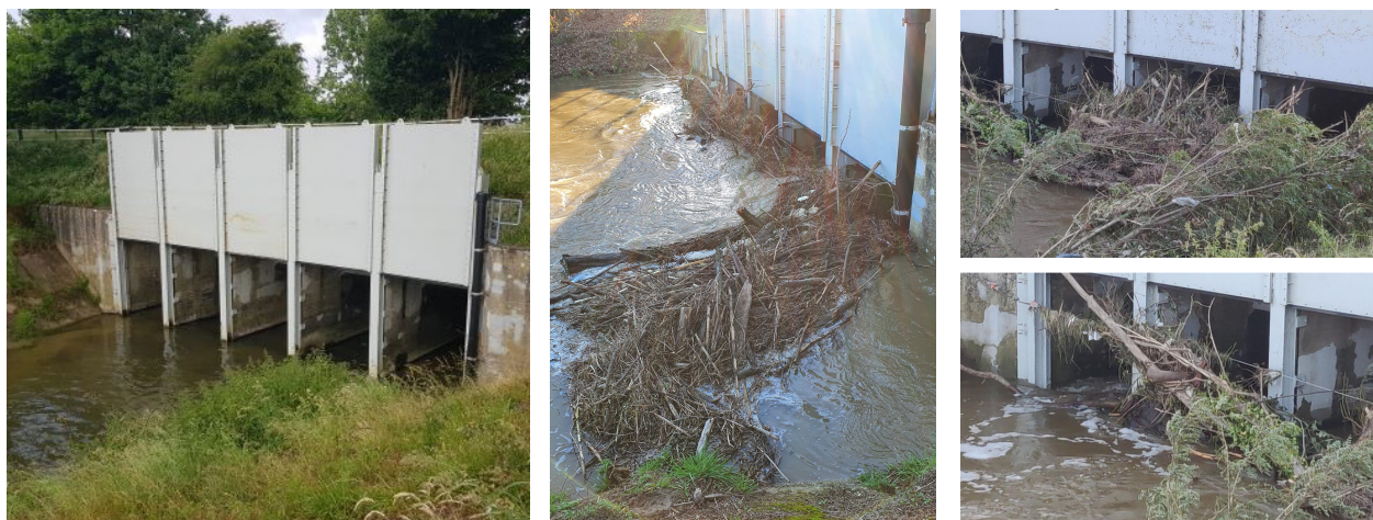
Figure 1. Inverted siphon near Bunde (the Netherlands), affected by driftwood accumulation during the summer 2021 flood. Credit rightmost photos Waterschap Limburg.
